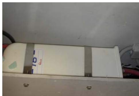
Hot water tank
