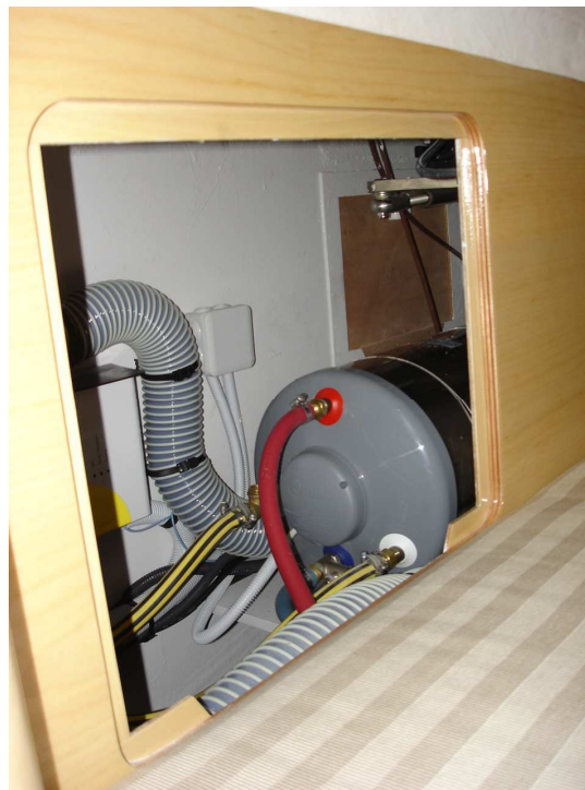
Location of technical room beneath cockpit
